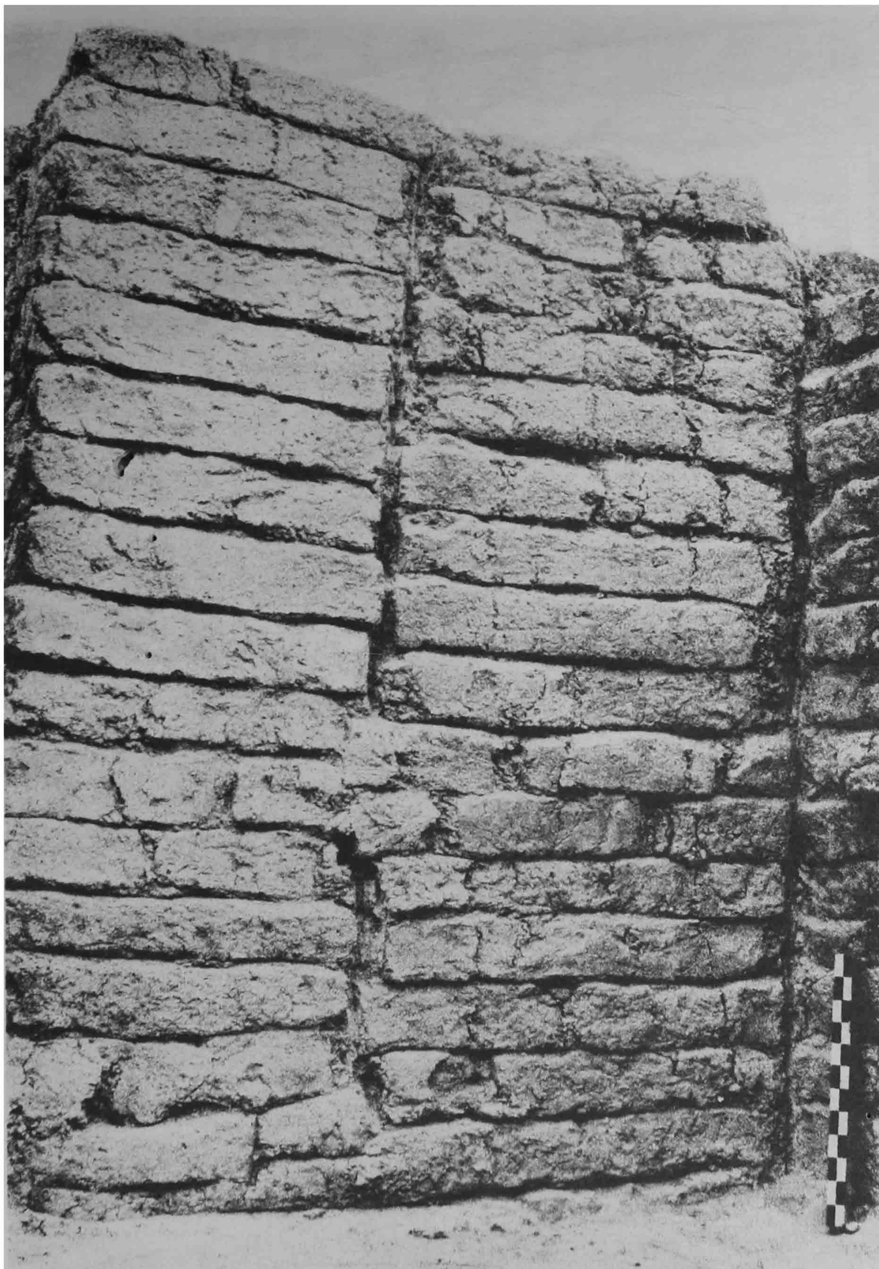
Two adjacent walls of structure showing the weak bonds of brickwork, KKG 2.
