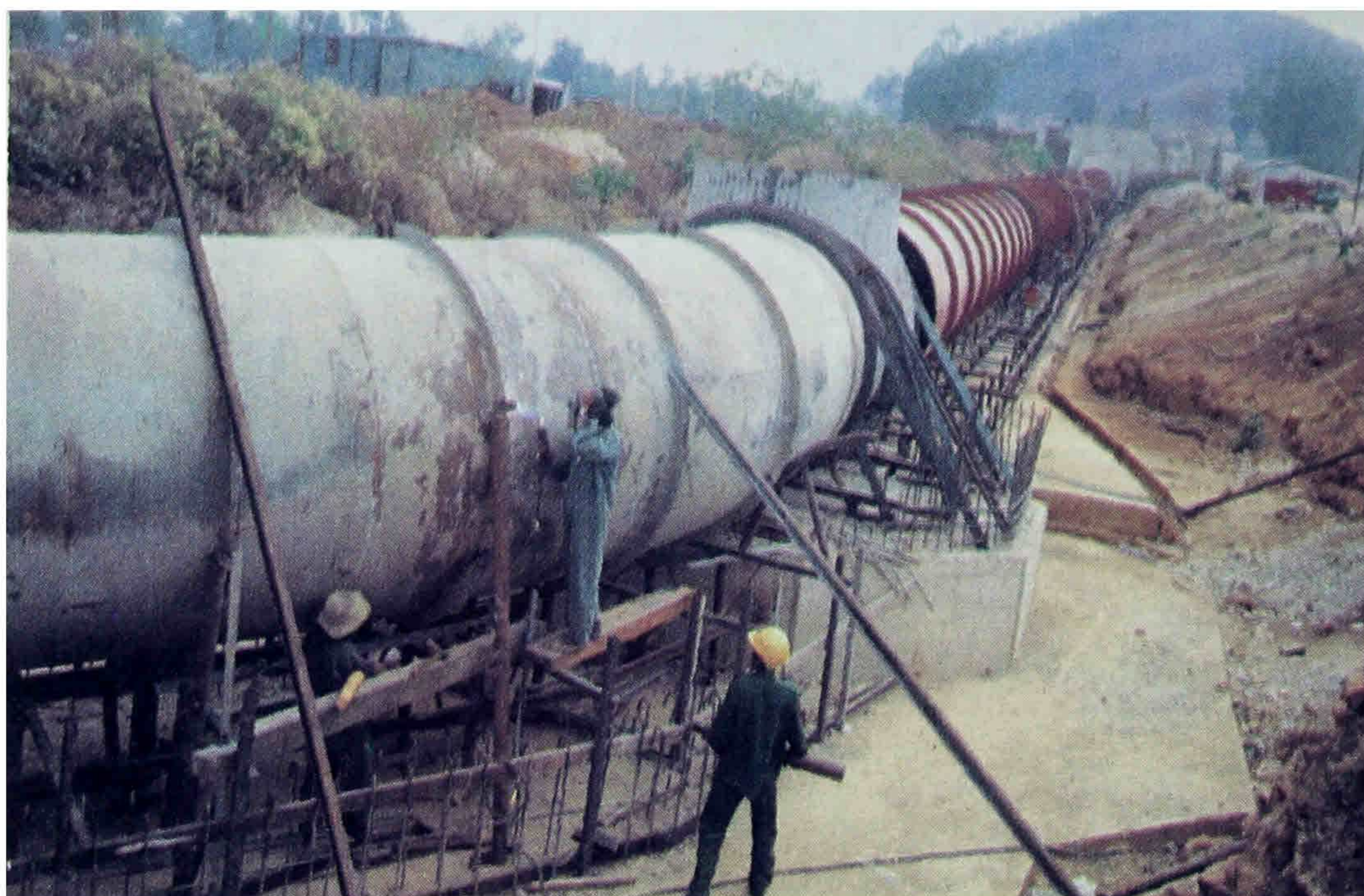
Zawgyi Electric Power Station Pipeline
